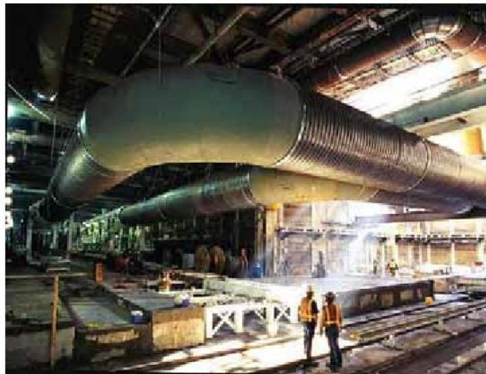
Figure 4-19: Underground Ventilation Ducts
