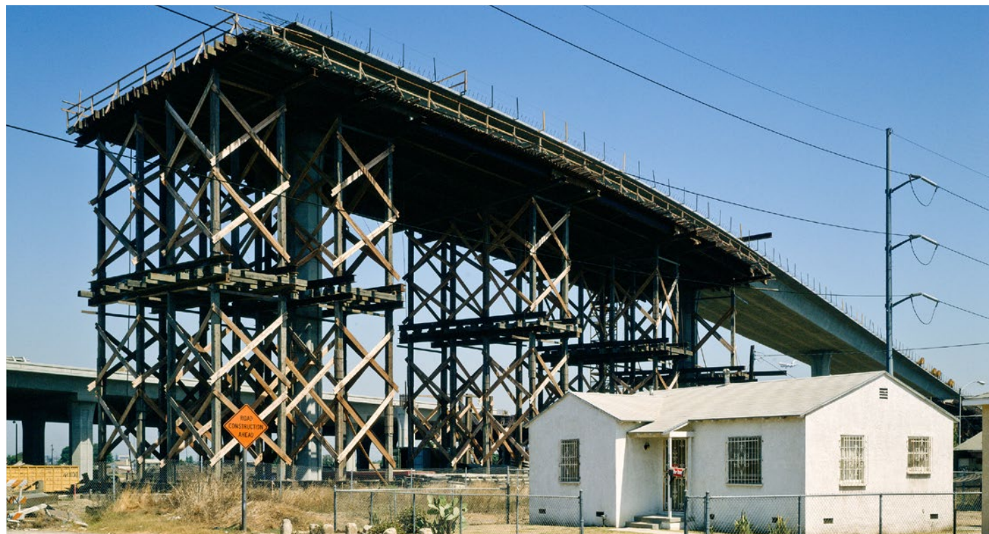
Source: John Humble. Construction of I-105 on-ramp in Lennox neighborhood of LA County.
