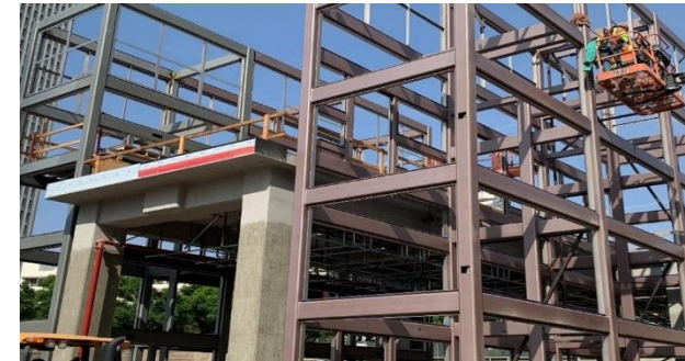
Welding for elevator hoist way frames at Grand Av Arts/Bunker Hill Station
