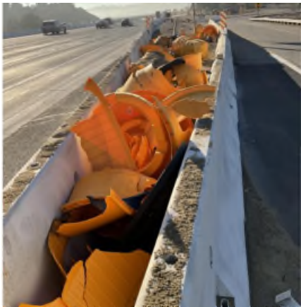
Damaged crash cushion from accident during holidays
