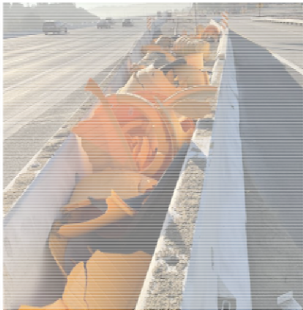
Damaged crash cushion from accident during holidays
