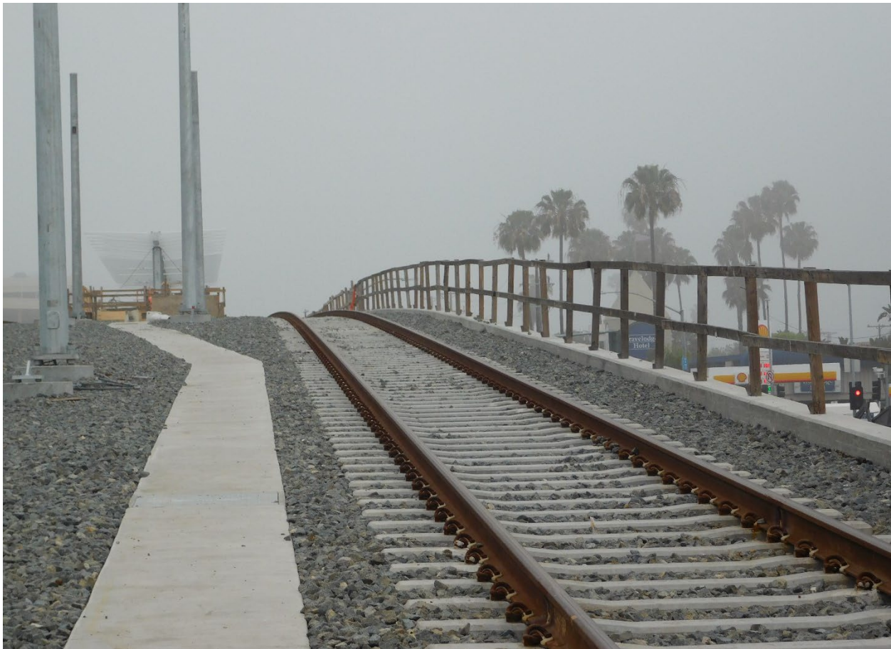
Crenshaw project – K Line - Elevated rail above Aviation Blvd. and W. Century Blvd.
