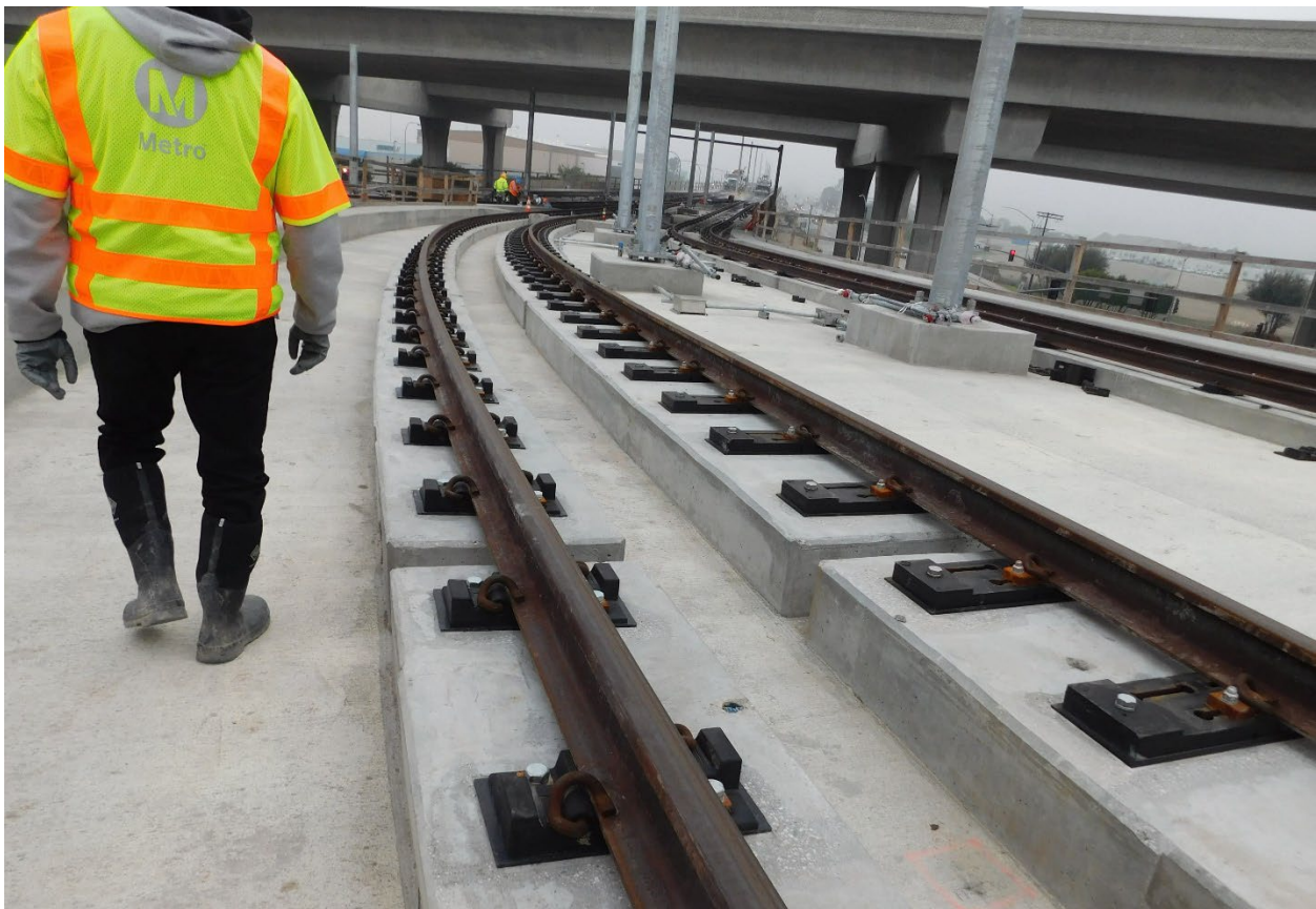
Crenshaw project – K Line - Elevated concrete fixed rail above Imperial Highway and below 105 Freeway
