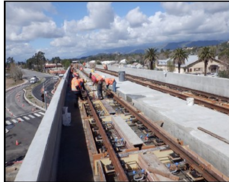
Bonita / Cataract – Structure Track Direct fixation
