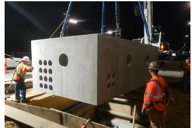
Installation of 1 of 4 vaults by W.A. Rasic on Van Nuys Blvd, between Vanowen and Vose.
