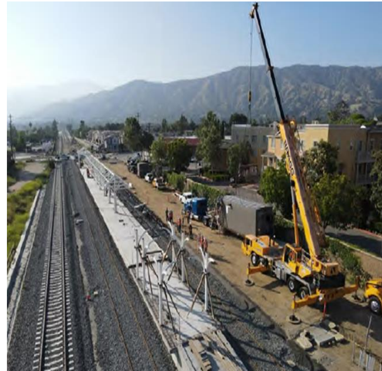
Glendora Station – Communication Bungalow
