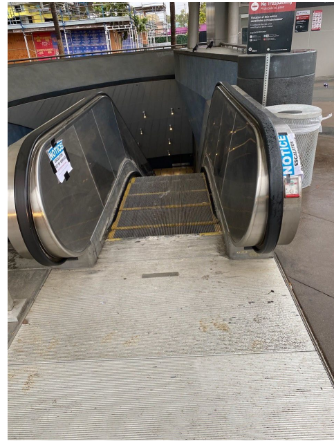
Escalators were shut off at 5 stations for safety reasons
