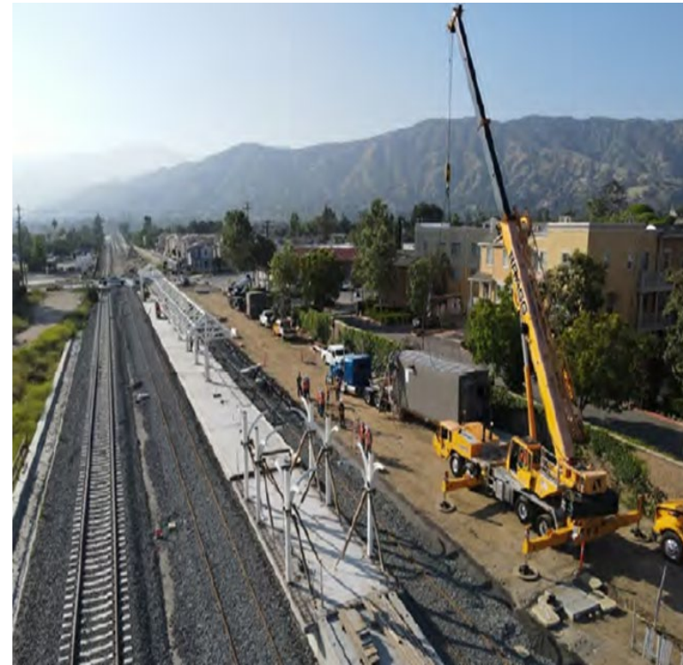
Glendora Station – Communication Bungalow
