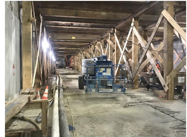
Century City Constellation Station Falsework for 2 nd level wall construction at east end
