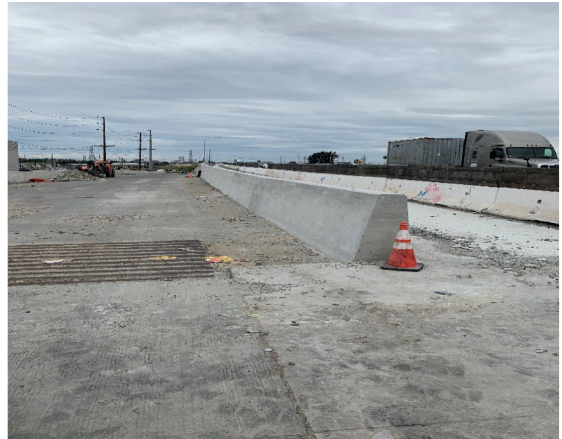
NB Crenshaw Blvd to SB 405 on ramp (RW#803) completed concrete barrier slab (Looking North)
