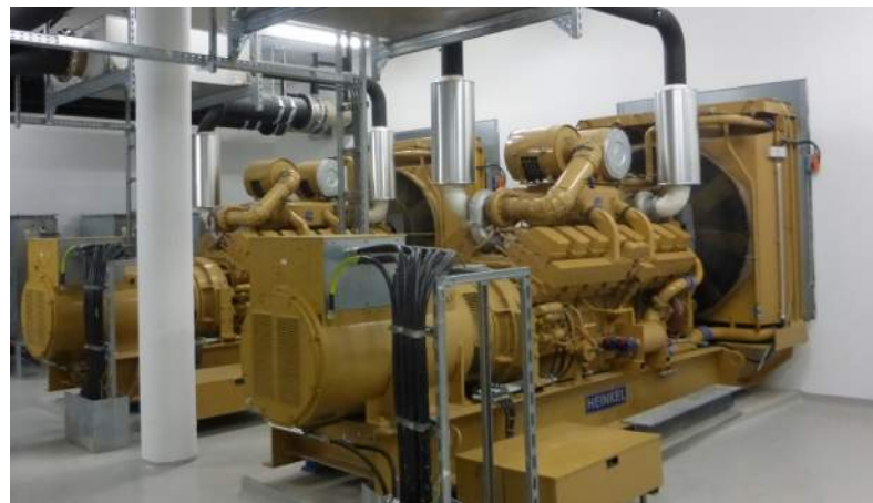
Image 43 – Backup Power Generators
