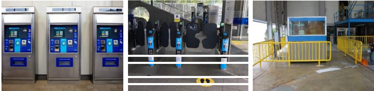
Image 44 – Examples of Access Control and Ticketing
