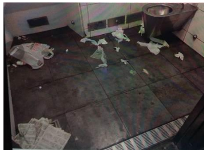
LEFT & RIGHT: Persistent vandalism in/around traditional restrooms, trash fires, and inaccessible elevators at El Monte
