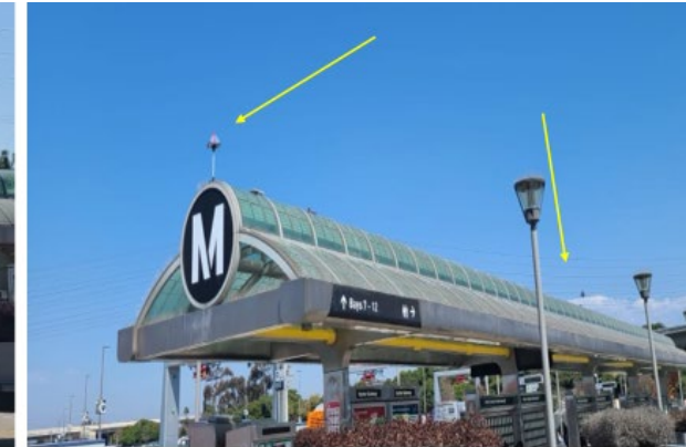
East Canopy – Device INSTALLED
