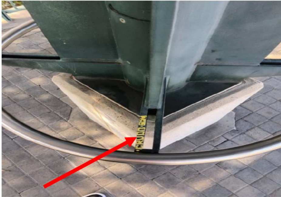
Lincoln/Cypress Station: 2024A-002 July 30, 2025 - Graffiti
