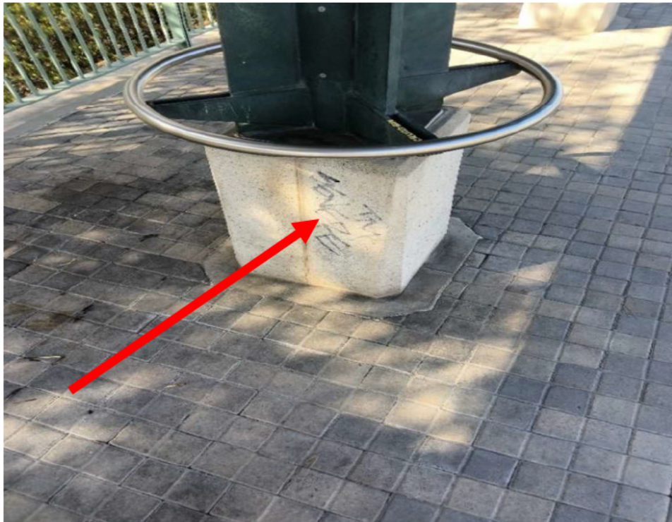
Lincoln/Cypress Station: 2024A-003 July 30, 2025 – Graffiti
