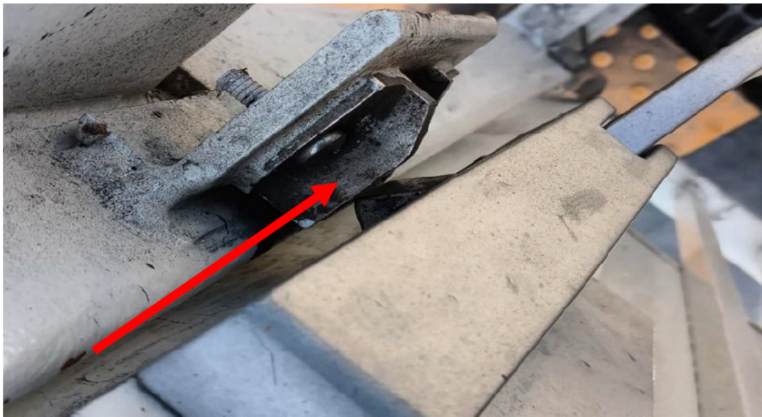
Leimert Park Station: 2024K-001 July 29, 2025 - Broken Latch
