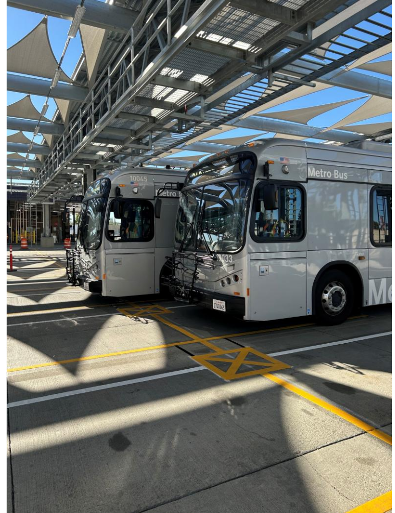
Buses at Division 9 Charging Station
