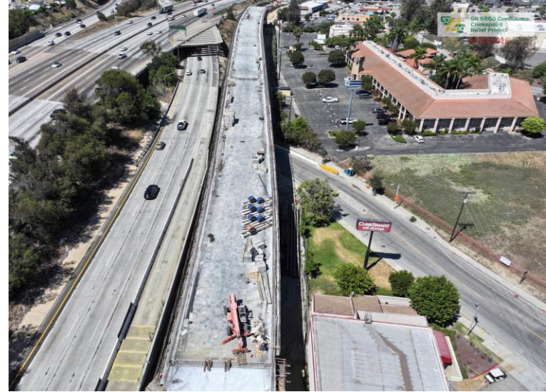
Bent and Hinge work at EB 60 Bypass Viaduct
