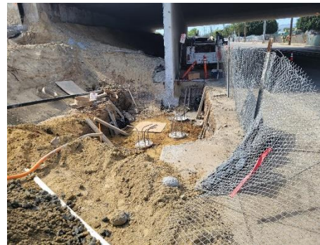
NE side of Van Ness Ave Bridge Widening showing CIDH for footing – looking South
