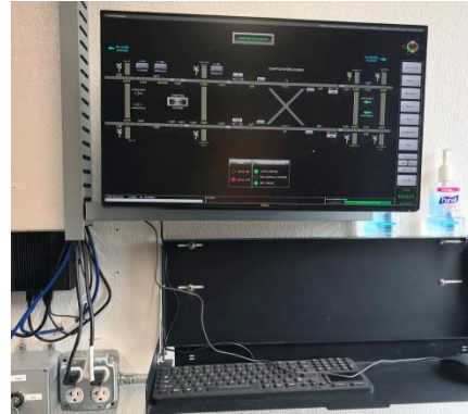
New Compton Interlocking Local Control Panel (LCP)
