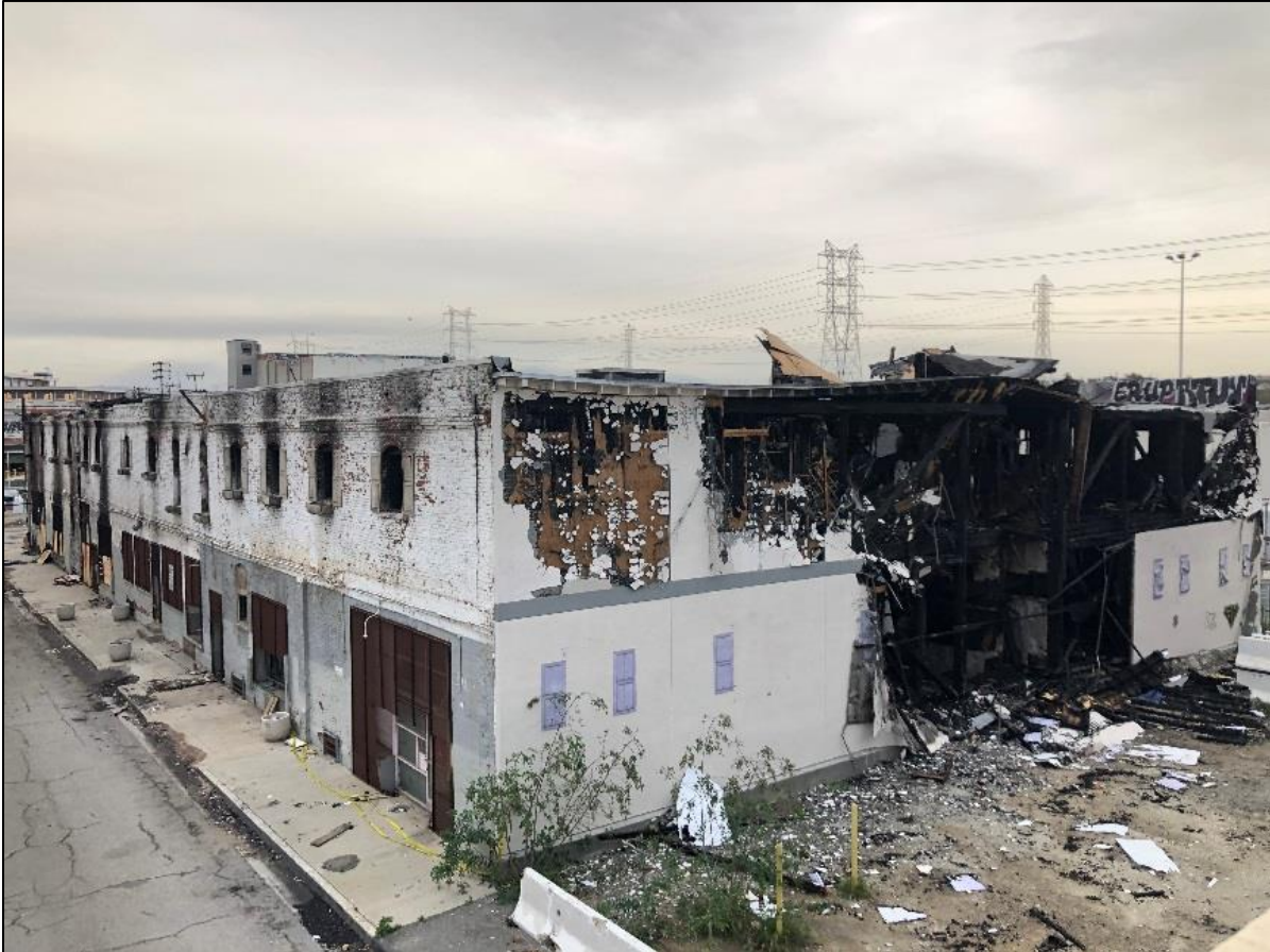
Figure 11. Citizens Warehouse/Lysle Storage Company (Pickle Works). West and south elevations. Looking northeast. ICF: November, 2018.
