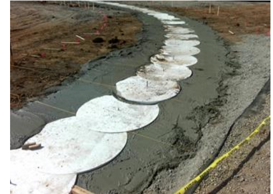
First 100 ft. of TTES Guide Wall Placement at Western VA Staging Area
