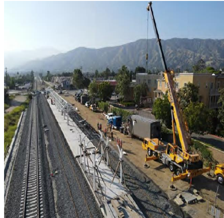
Glendora Station – Communication Bungalow
