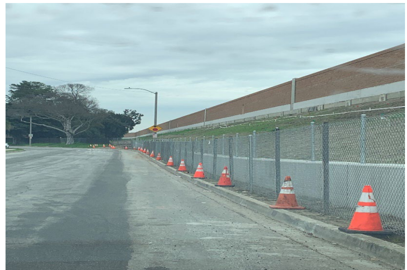
NB 405 South of Van Ness Blvd (SW #760) with completed retaining concrete barrier at 186 th Street
