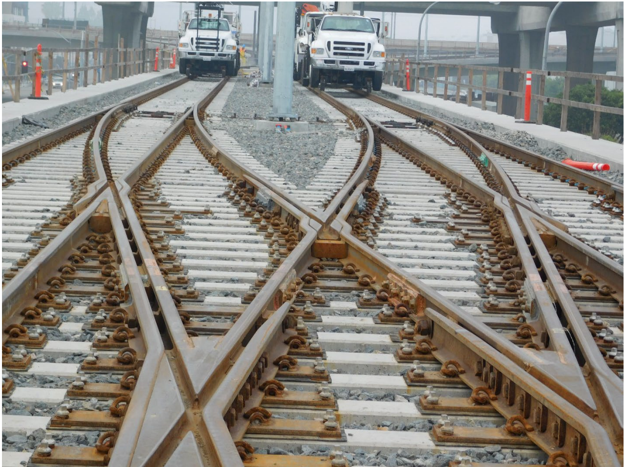
Crenshaw project - Elevated double crossover rail above Aviation Blvd. and below 105 freeway
