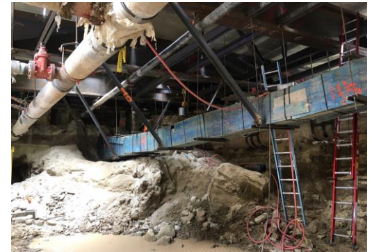
Utility Hanging Under Constellation Blvd.
