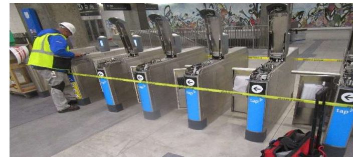
MLK Station – Performing configuration programming and software testing to TVM and fare gate system
