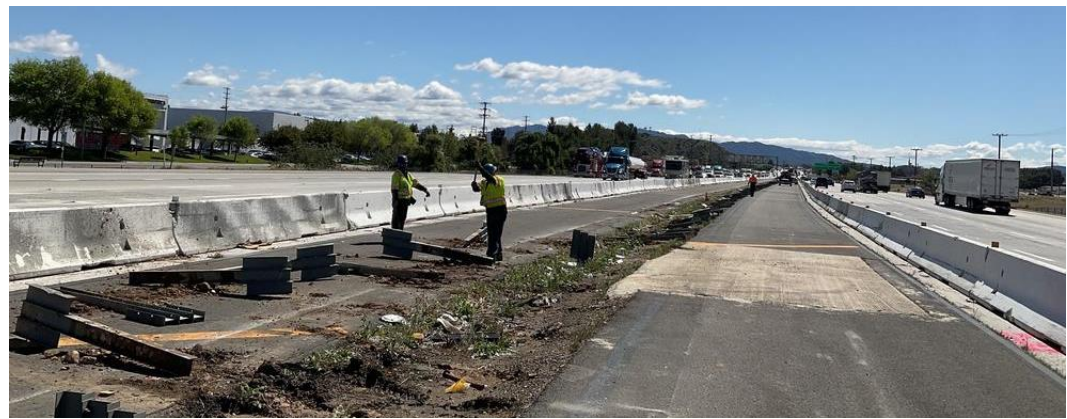
Removal of existing metal beam guardrail from median – Rye Canyon Road to Parker Road
