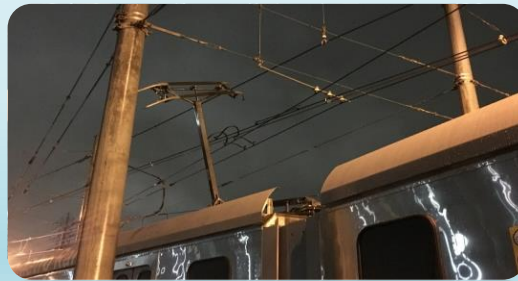
(5) Pantograph Entanglement with OCS Wires
