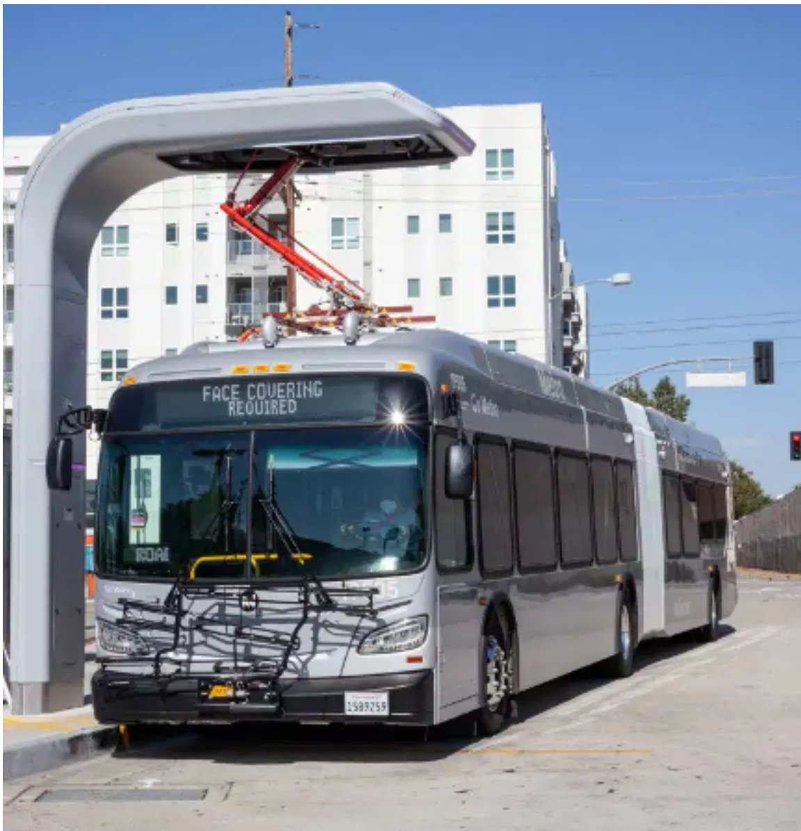
Figure E.2-1. North Hollywood Station On-Route Charger
