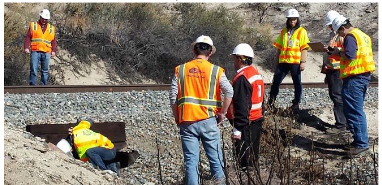
Picture 2: SCRRA Staff and MTA Staff Inspecting a Wood Box Culvert on the Valley Subdivision
