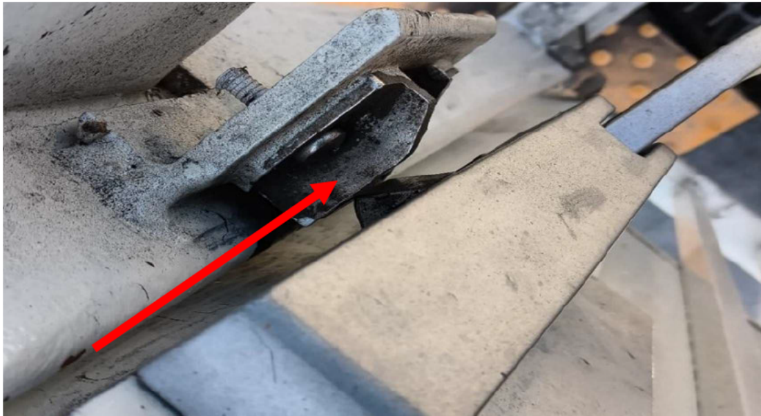
Leimert Park Station: 2024K-001 July 29, 2025 - Broken Latch
