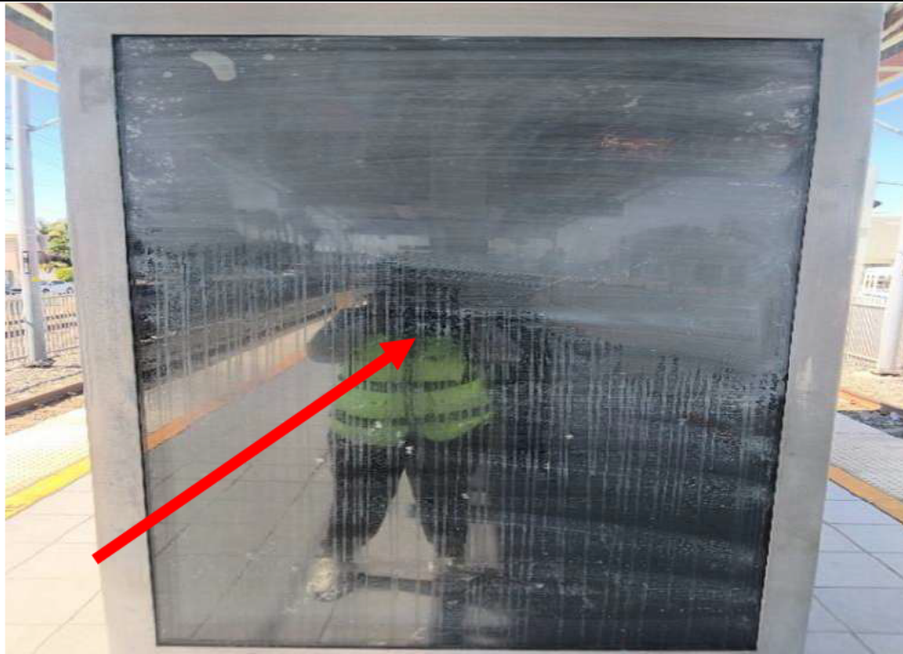
Compton Station: 2024A-007 July 30, 2025 - Damaged Map Case
