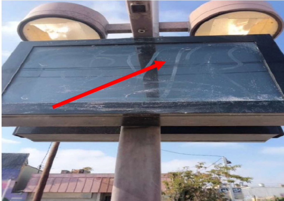
Pico/Aliso Station: 2024E-001 July 29, 2025 - Broken Monitor
