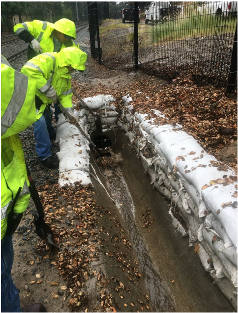
Flood prevention near tracks to avoid service disruption
