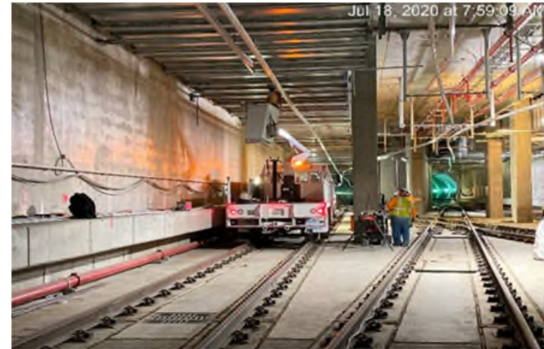
Continue installing supports and fixtures for the crossover lighting at the invert level of Expo/Crenshaw Station.
