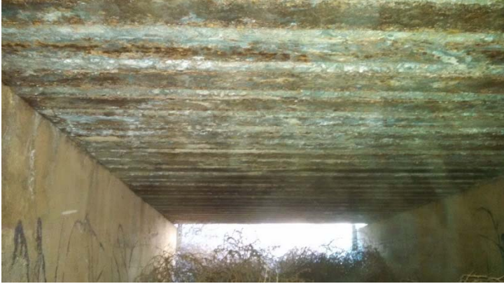
Picture 5: The inside of one of the top 3 Priority "Rail-Top" Bridges on the Valley Subdivision
