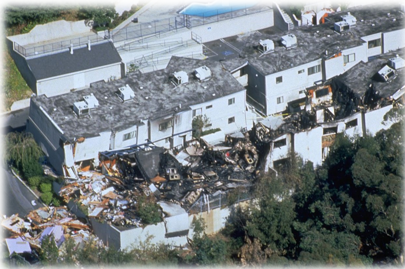
Caption: Soft Story Building Collapse at Northridge, California.
