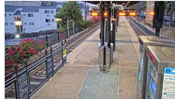
New upgraded cameras at South Pasadena Station (left) and Southwest Museum Station (right)
