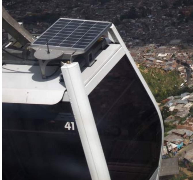
Image 37 – Solar Panels Mounted to Cabin Roof
