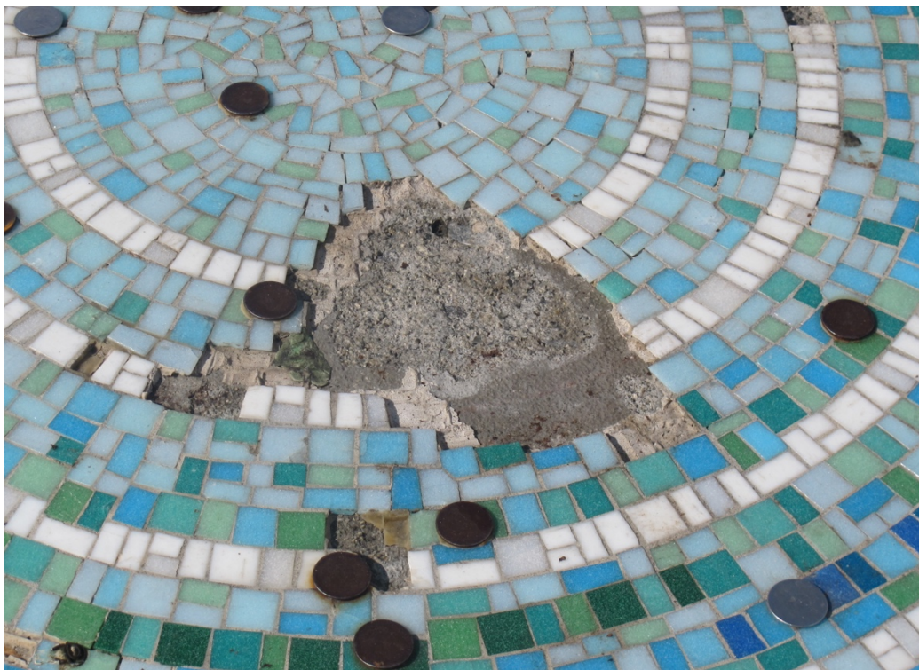
Metro Blue Line – Damaged artwork mosaic tile requires specialized repairs
